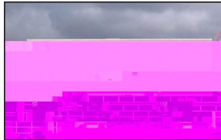
The roof of the gym indicates an attempt to use standard campus architectural vocabulary on a large flat roof structure. Window and column forms recall those used on classroom buildings.
